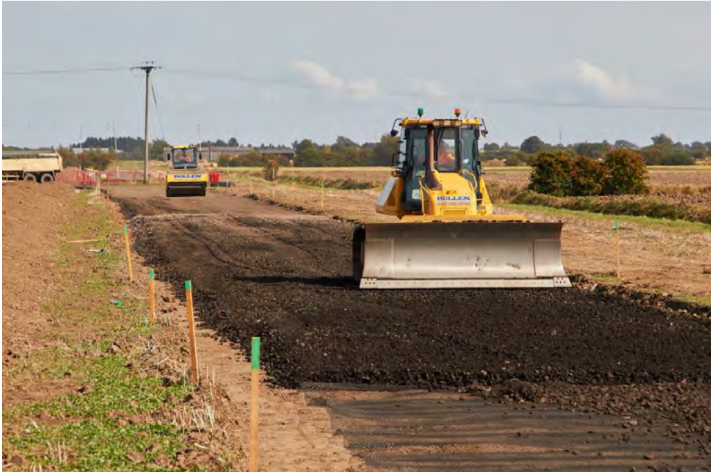
Plate 3.1 Indicative haul road construction with a bulldozer in the foreground (right) and a roller in the background (left) (Source: Siemens, 2018)
