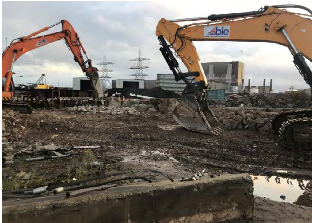
Plate 3.2 Indicative yellow plant with a bucket (right) and a hydraulic breaker (left) used during construction of Triton Knoll (Source: RWE, 2020)
